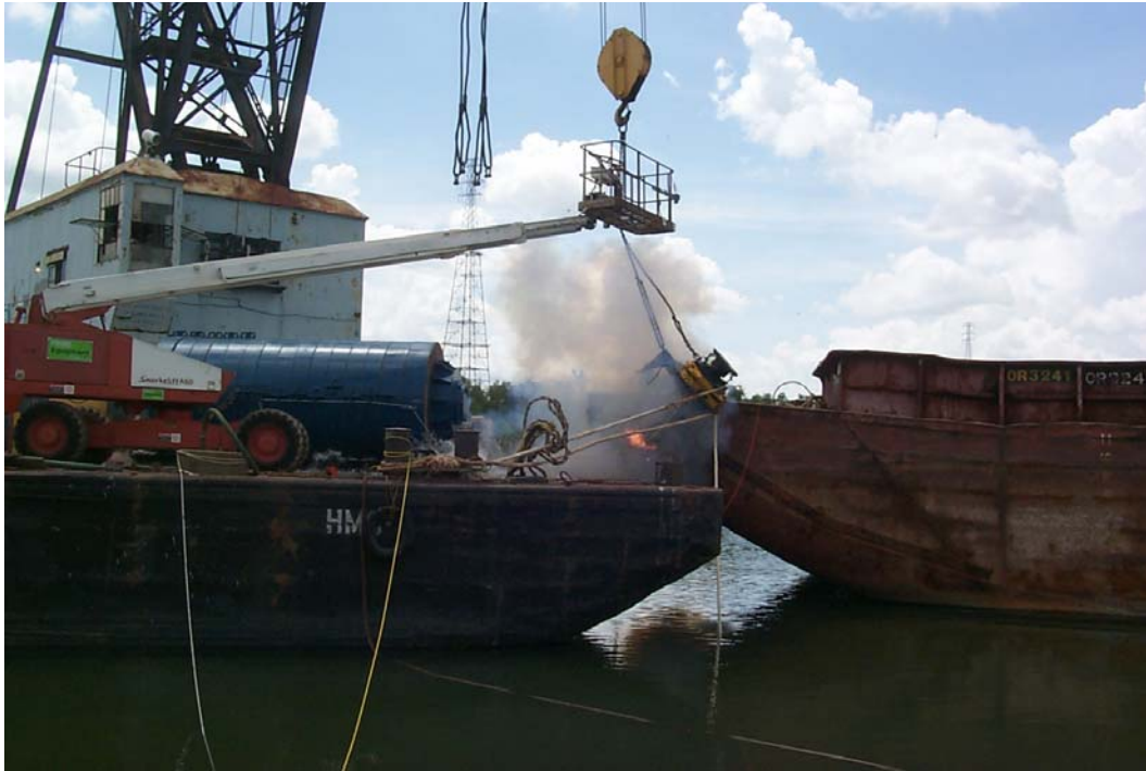
Figure F-3. Statnamic device and experimental setup during experiment (Note: The detonation of the Statnamic device has just occurred at the time of the photograph)
